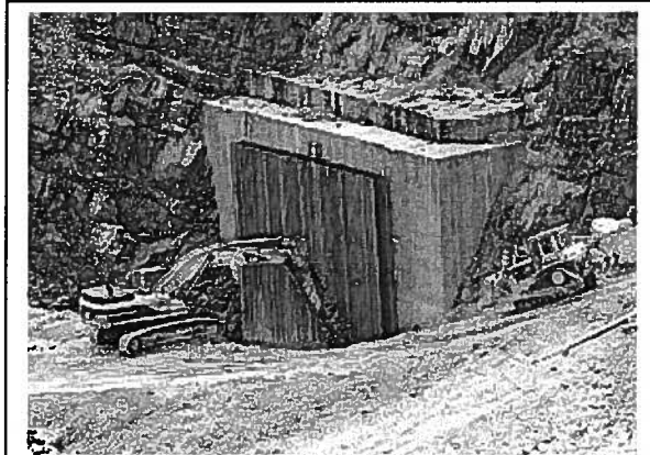
Steel beams have been placed at the entrance to the half-mile long American River diversion tunnel, which has piped the waterway underground since the early 1970s. The channel has been restored and boating will be allowed again early next year. Photo by Ben Furtado/Auburn Journal
