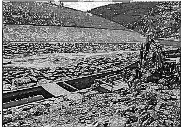
With the American River re-channeled and the Placer County Water Agency's permanent pump station in place, work is nearing completion on the $75 million project in the canyon below Auburn. Photo by Ben Furtado/Auburn Journal
